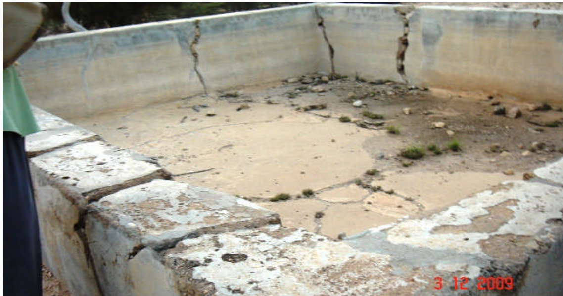
Broken water reservoirs Dabis River (GWX)
